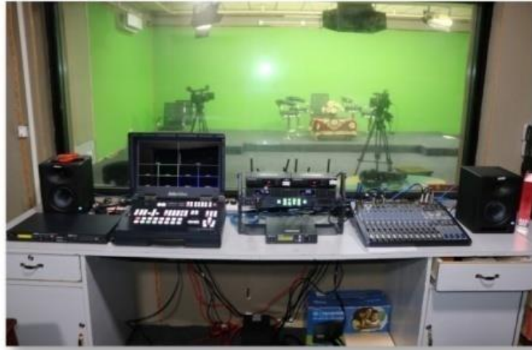
PRODUCTION CONTROL ROOM (PCR) EQUIPPED WITH H5 1300 DATA VIDEO SWITCHER HDR 70 RECORDER, AUDIO DELAY BOX , PRESONOUS AUDIO MIXER AND STUDIO AUDIO MONITORS
